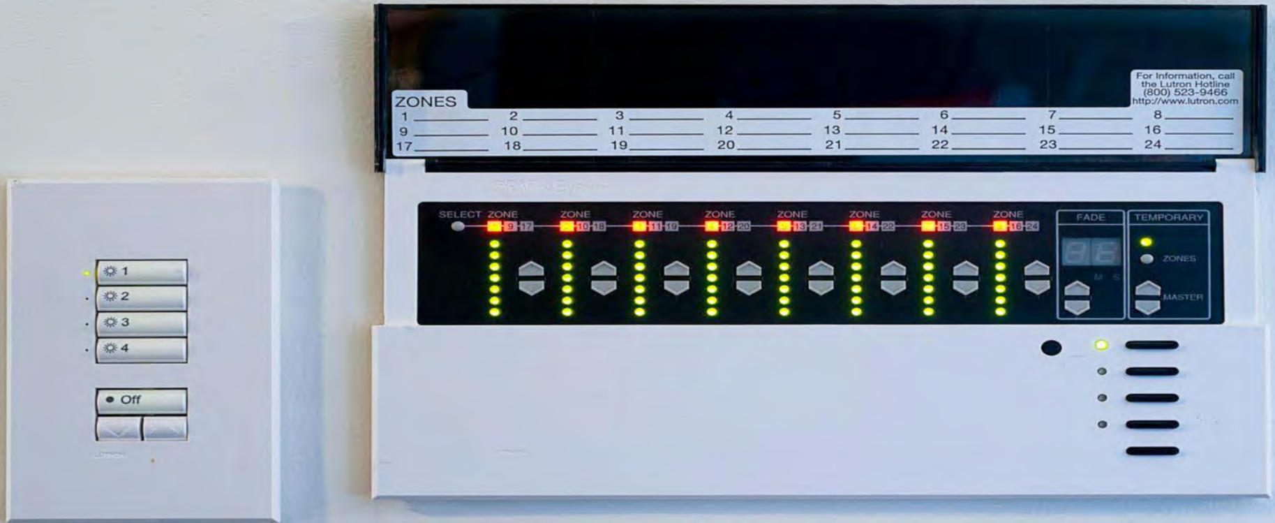
Commercial lighting control panel in the modern (2010) Media Lab Building
